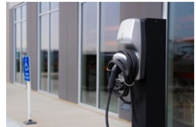
Five EV charging stations are available for customers and Vallen associates.
